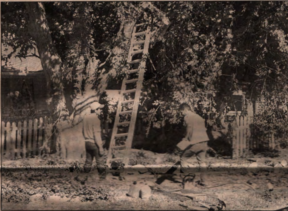
After high winds swept the area recently, workers prepare to remove a damaged hackberry tree located in front of Salado Haus and Ambrosia Tea Room. The workers completed their task preventing any damage to parked cars.
