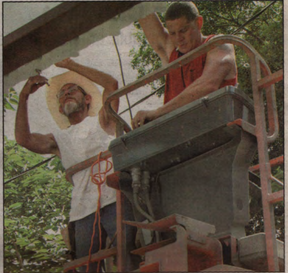
Richard Goodwin and Darin Crawford, of ERW Construction, attached metal siding on the Church of Christ Youth Center, now under construction on Church Street. (PHOTO BY TIM FLEISCHER)
