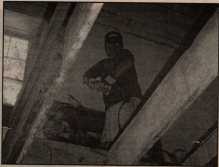
Chris Kimber peers through beams of the second-story floor. (photo by John Eubanks)
