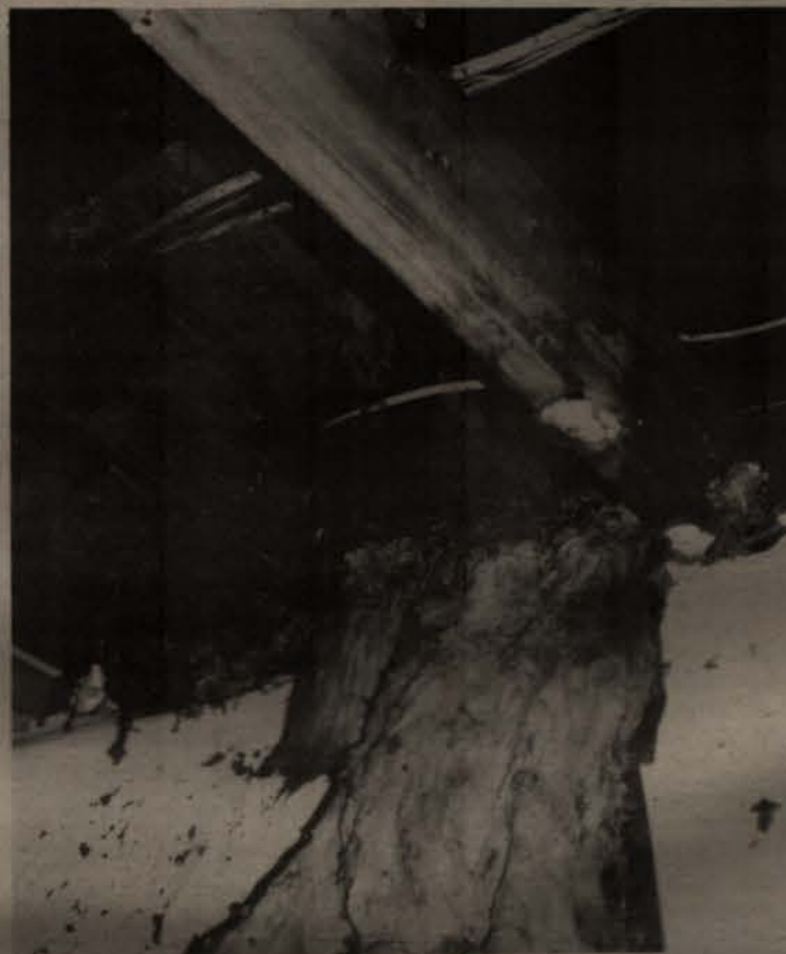
Burned insulation in the attic of the Stagecoach Inn hotel is shown above. The hotel caught fire Oct. 9 with damage to 15 rooms. (photo by John Eubanks)
