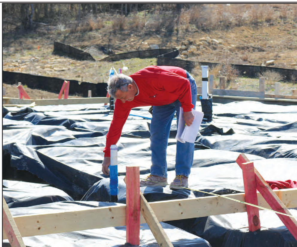
Kenny Christianson with Christianson Plumbing and Air Conditioning checks his plumbing work on a house pad at Meadow Crest Dr., which connects Royal St. to Hester Way. The addition in Mill Creek Springs is being built by Emerald Homes, a division of DR Horton Homes. (PHOTO BY TIM FLEISCHER)
