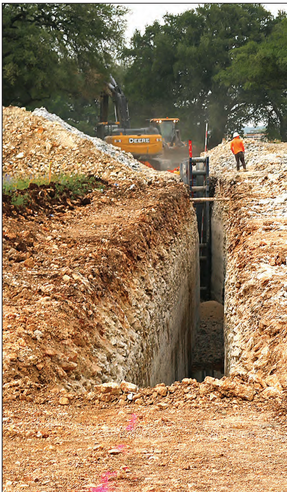
(PHOTO BY TIM FLEISCHER) Excavating the trench for sewer lines at Water's Edge.
