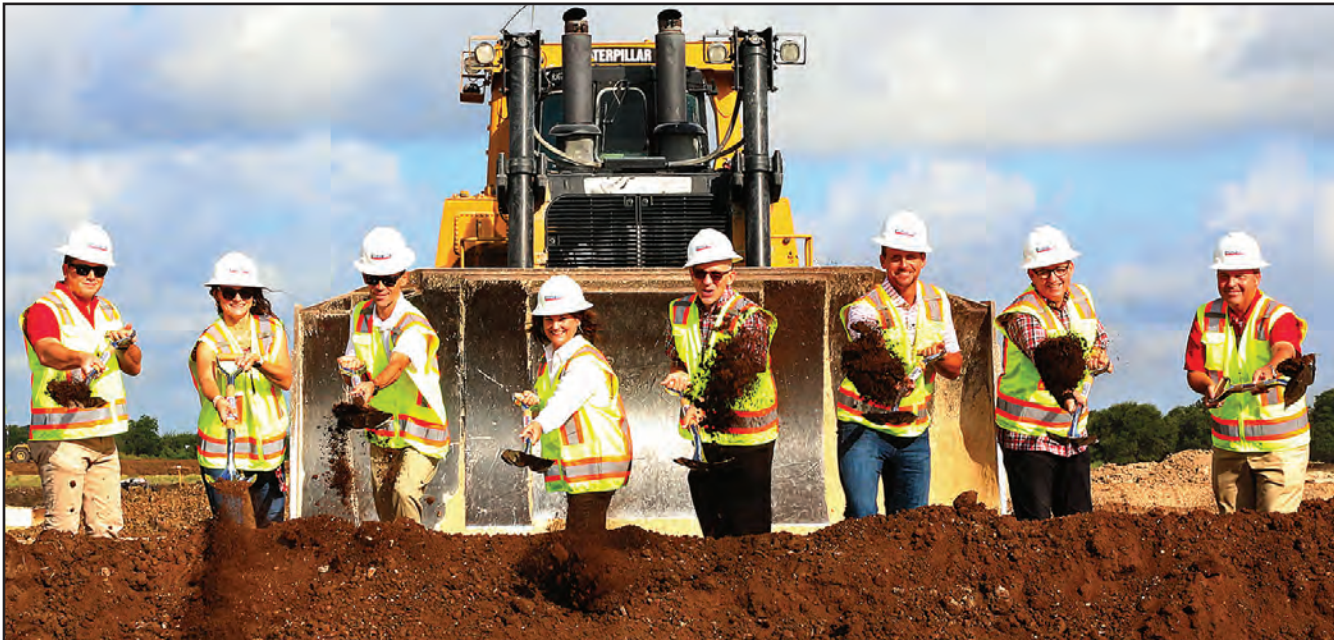
Salado ISD broke ground on the 250,000 sq. ft. high school on July 29. Shown above, from left, are SISD Trustees Cooper Gill, Savannah Hennig, Chris Diem and Amy McLane, SISD Superintendent Michael Novotny, Trustees Eric Malmin and Jim Reed and State Representative Brad Buckley. (PHOTO BY ROYCE WIGGIN)
