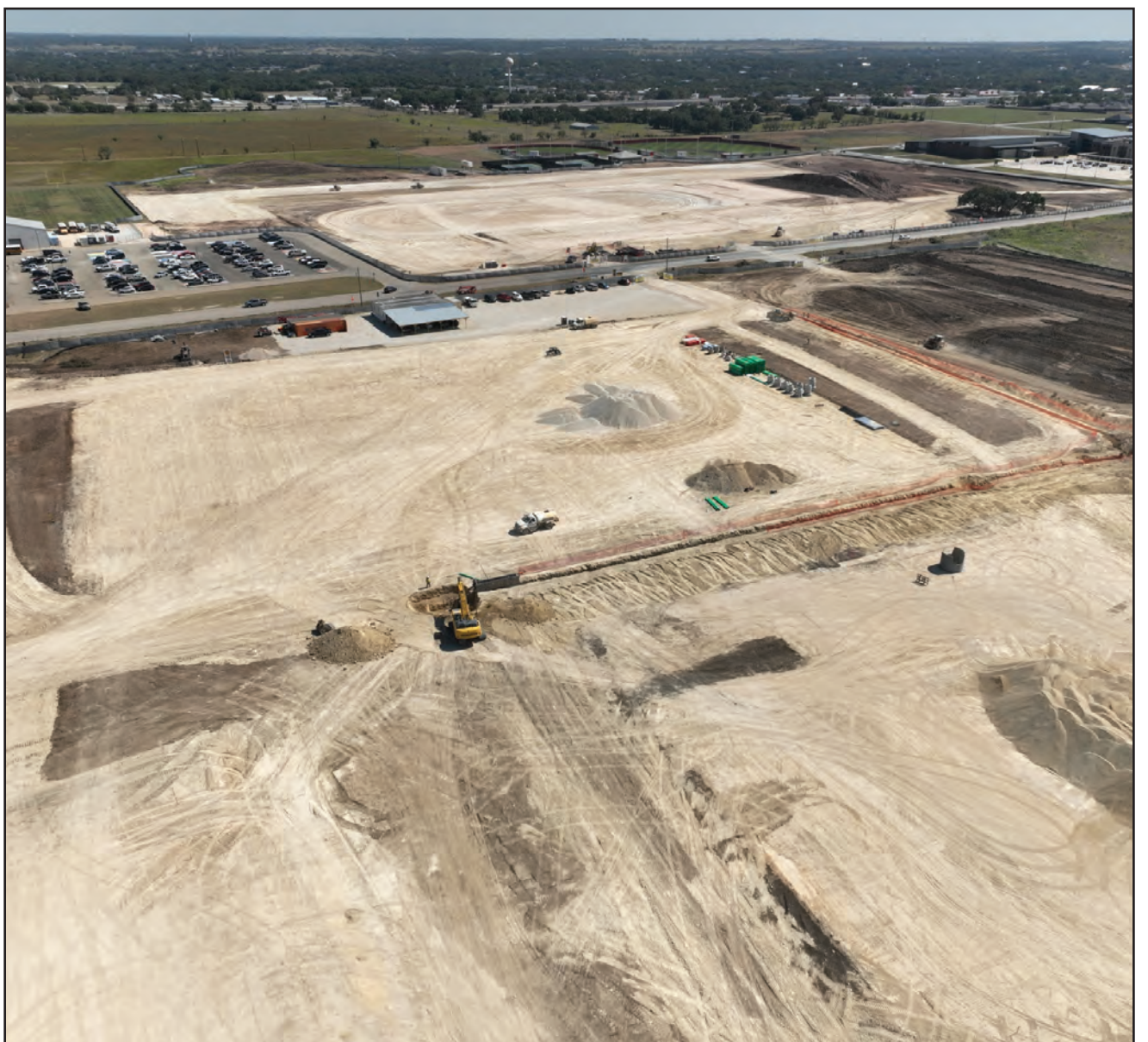
Aerial of work at the new Salado High School campus. (COURTESY PHOTO)
